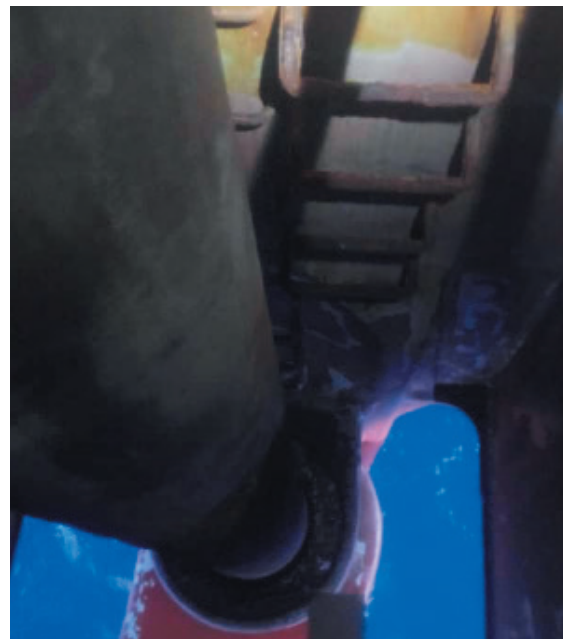
Image 2: Internal ladder housing
